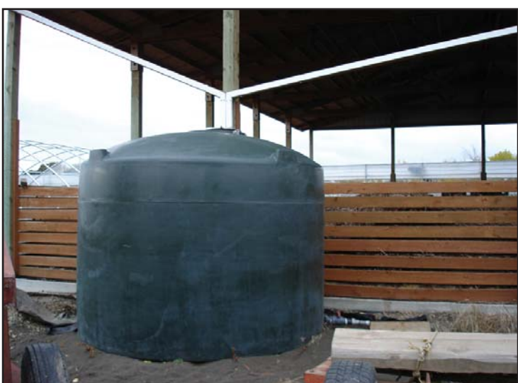
Rainwater storage tank
