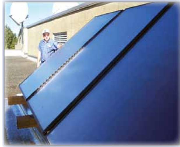
Hilmo Ljucevic checking solar panels on a campus roof
