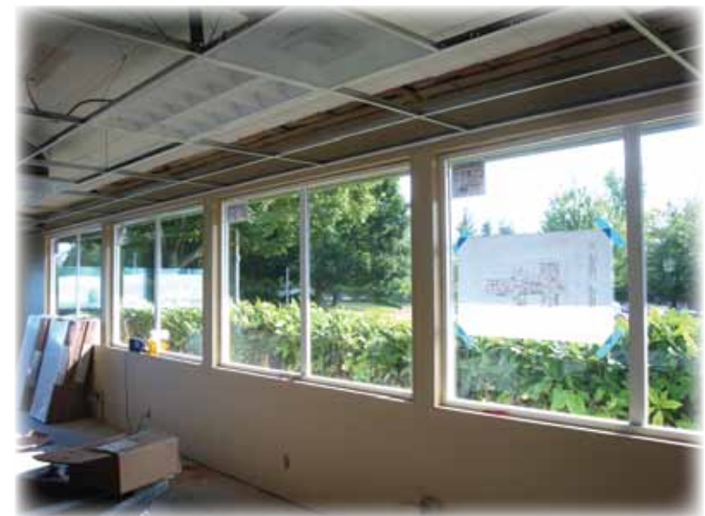
Old assessor's building gets new energy-efficient windows in preparation for new occupants.
